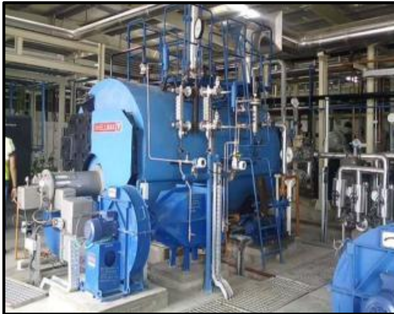
Propane Fired Boiler (New)
