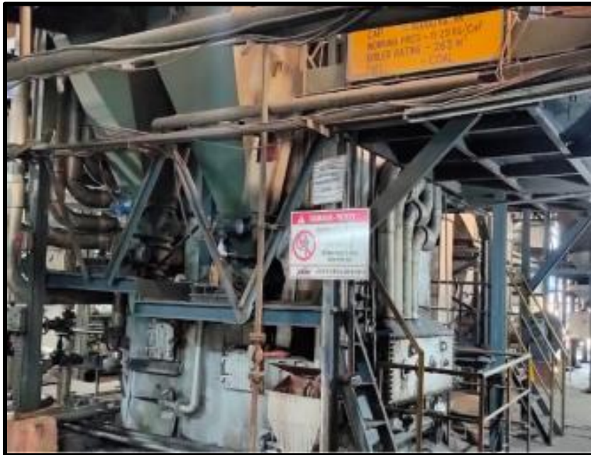
Coal Fired Boiler (Existing)
